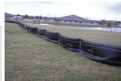
Silt fence installed backward, with no trenching. "Decorative"
