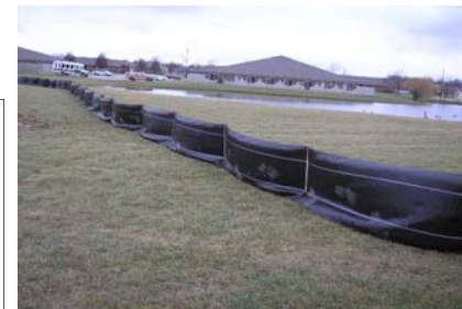
Silt fence installed backward, with no trenching.
